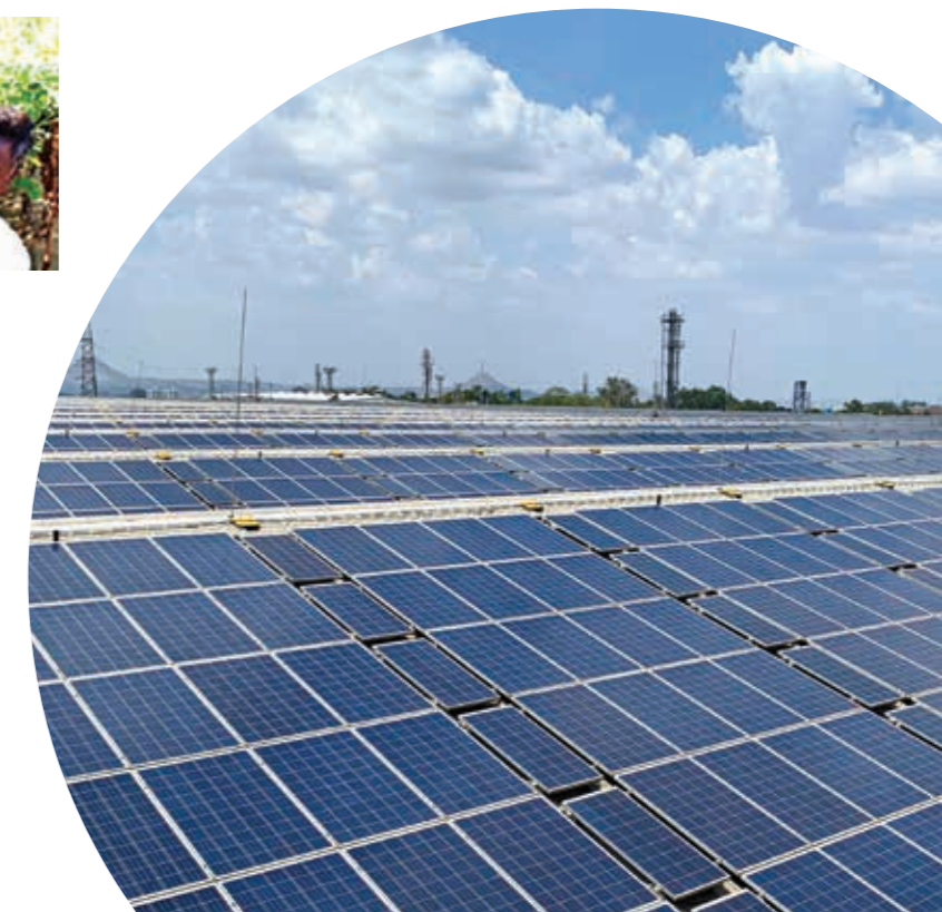
Roof top solar at Nashik plant
